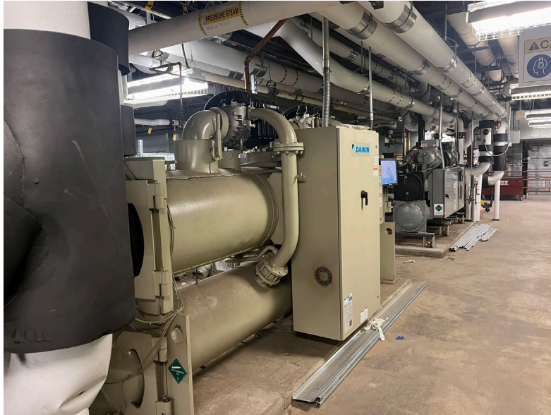
Figure 6: Interior of mechanical room in the Center of Science and Technology.
